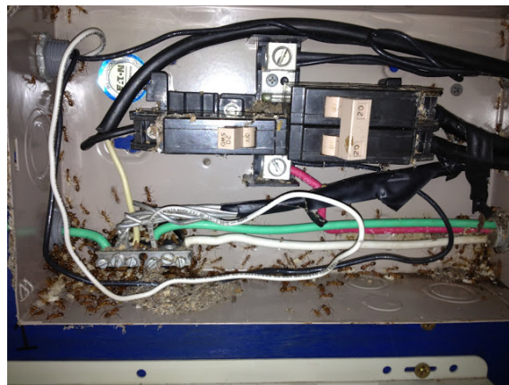
Figure 7: Invasion of the fuse box by ants that led to the failure of the solar controller in June 2012 Photo courtesy of Bryan Ferry
