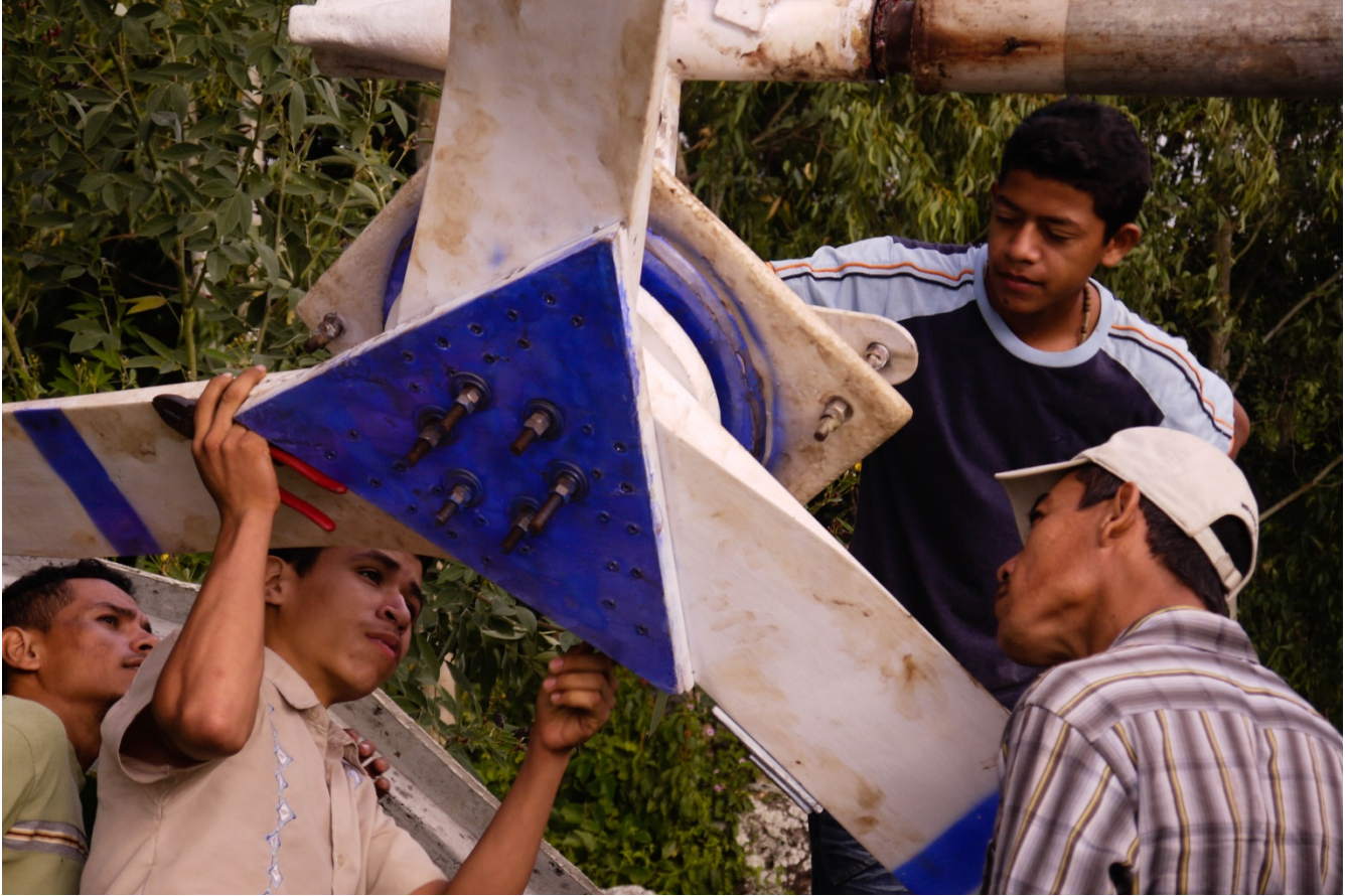
Figure 11: Inspection of the rotor and stator by the Cuajinicuil technicians to prevent potential future failures
