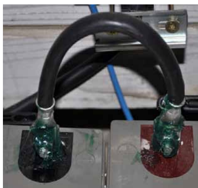
Fig. 56: Grease on connectors
