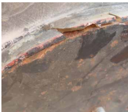
Fig. 33: Cracks in resin in the rotor edge
