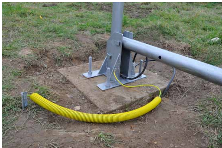
Fig. 2: Ground connection of the tower and electronics
